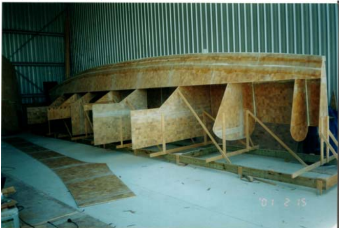
Full size hull panels are screwed in place. The join gaps are filled and the joins are taped.
