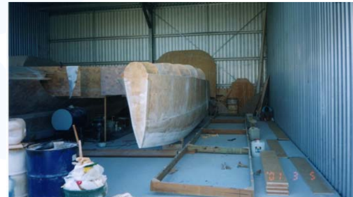
The hulls are joined with cross bulkheads, major cabin bulkheads, then the curved side decks are strip planked.
